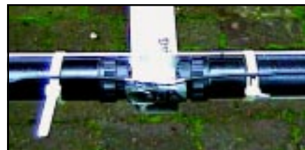
Here you can see the wires on the elements themselves.
